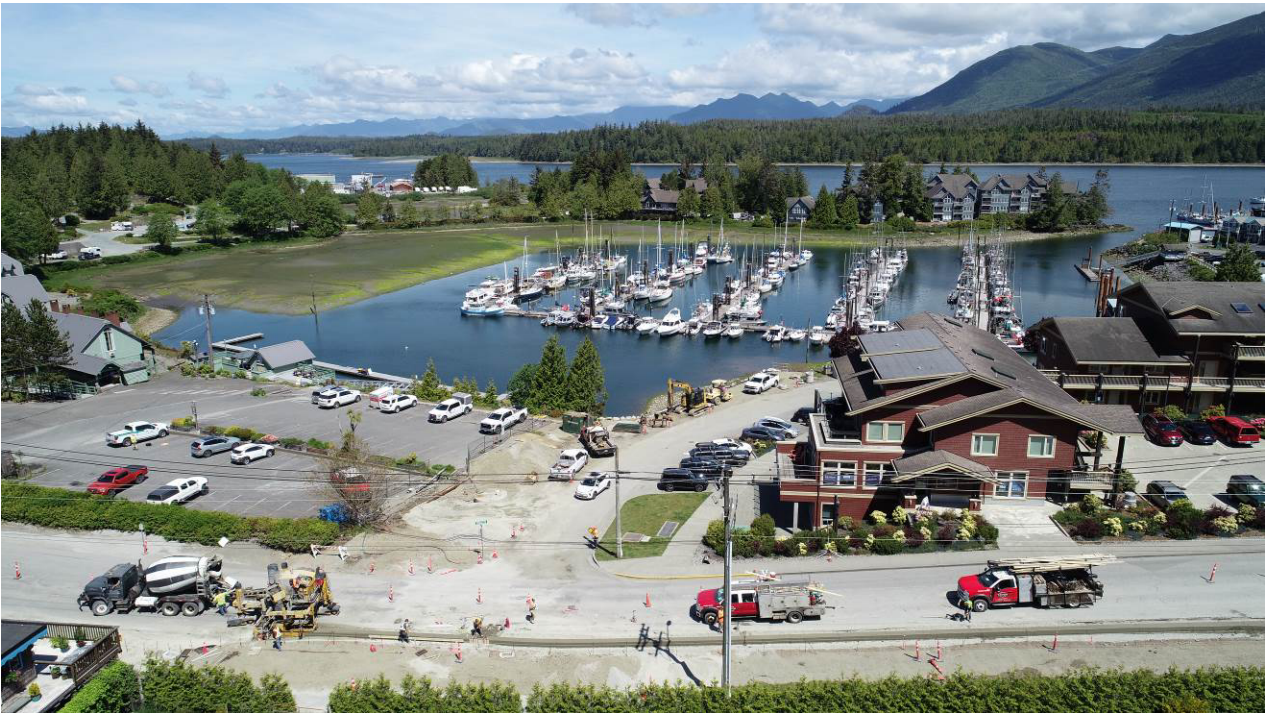
Photo #4 – Peninsula Road Curbing
