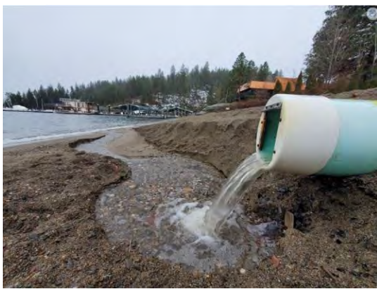
Figure 7. Uncontrolled stormwater outflow causing beach erosion.
