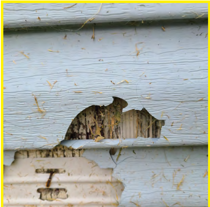
Photo 'B' above shows another location with the same issues as seen in photo 'A' to the left. The plywood wall sheathing is exposed and no building paper or weather barrier is seen which is a major building envelope assembly issue.
