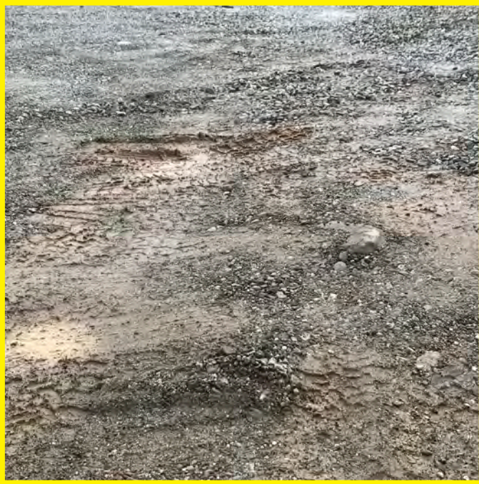
The photo above shows soft spots in the parking and training area of the site that become too soft to drive apparatus trucks over in the fall and winter months. Removal of soft areas and installation of structural fill materials is required in these areas.
