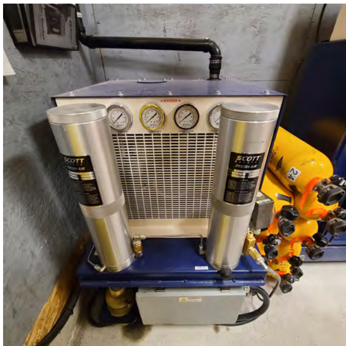
The photo above shows equipment that needs to be relocated to a proper clean environment.
