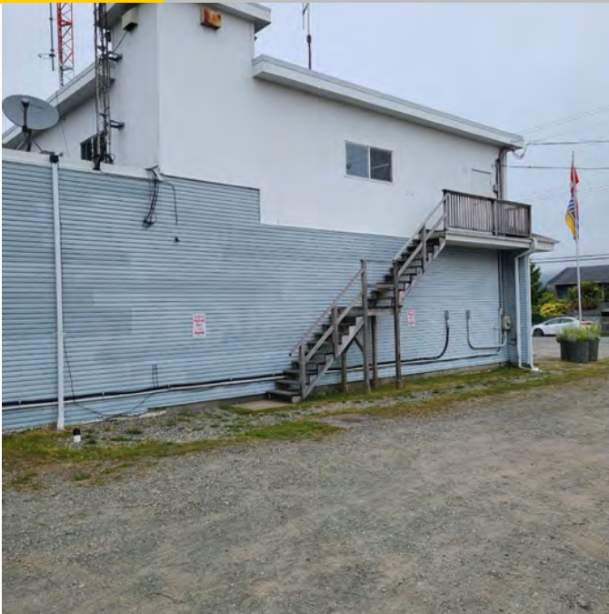
The photo above shows the patchwork of cladding materials and the only second level emergency exit staircase. Consistent lot deterioration is shown in this area as well.
