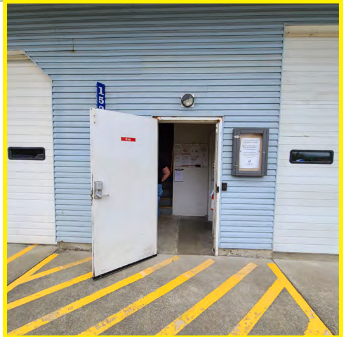
The photo above shows inadequate main entry lighting. The main entrance is not suitable for public access. Emergency egress (panic) hardware is not present.
