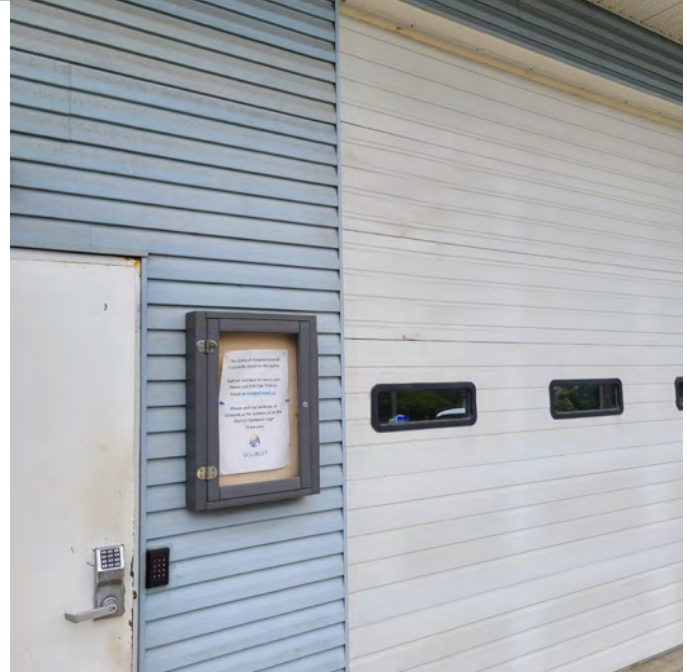
The photo above shows the main entry door and apparatus bay overhead doors. The doors and front facade have consistent wear and signs of weathering as the rest of the building. While the style of overhead doors are acceptable, they are too small.
