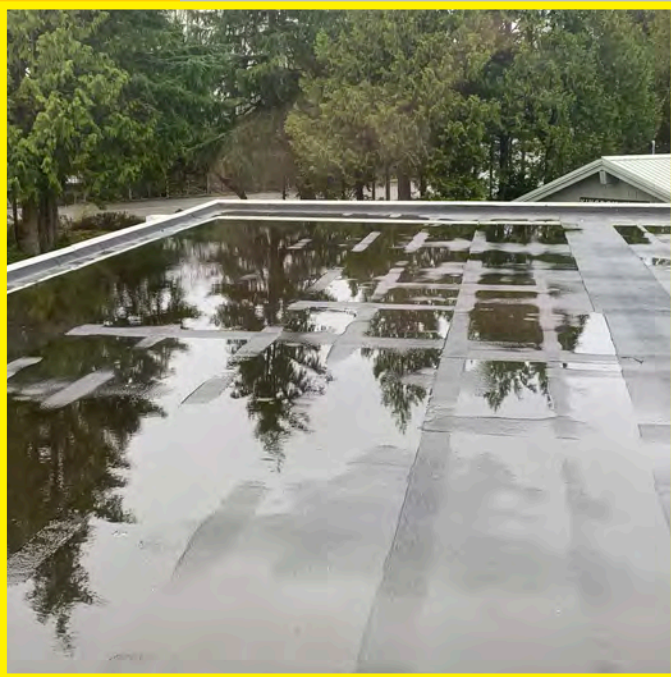
The photo above shows the general condition of the roof. The roof system is inadequately sloped causing water ponding during the fall and winter months. It is clear that the roof requires replacement.
