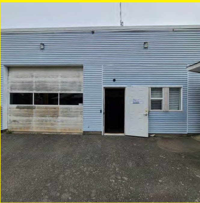
The photo above shows the overall facade deterioration and inadequate site lighting. Lighting should be upgraded to LED for energy efficiency. Windows and doors should be replaced for improved energy efficiency. No door panic hardware for exiting.
