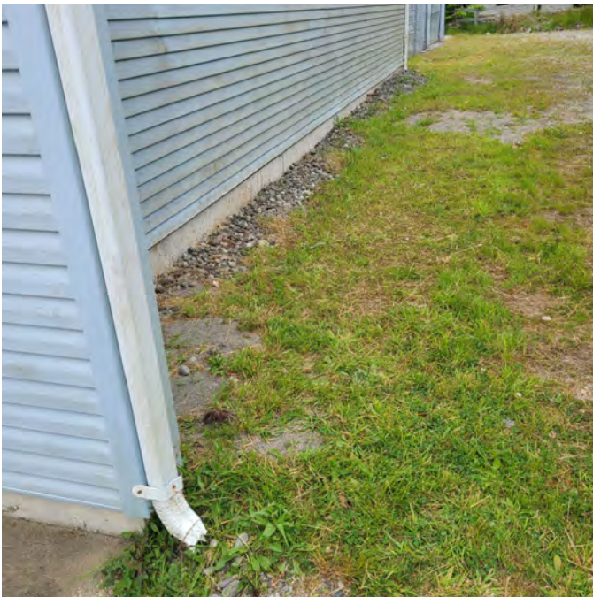
The photo above shows the overgrowth of organics are the site and lack of proper storm drainage. The site is not suitable for proper usage and training facilities. The current site conditions pose safety hazards to the public.
