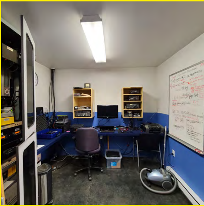
The photo shows an overall view of the EOC/ radio room.
