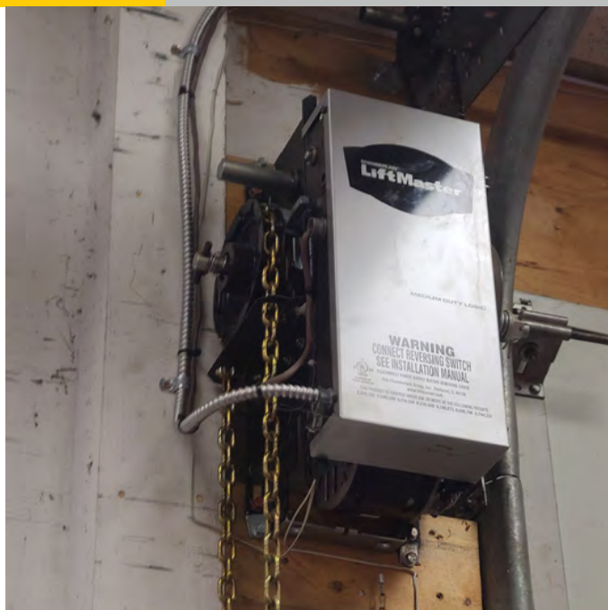
The photo above shows the existing Lift Master overhead door openers. Effective condition cannot be confirmed.
