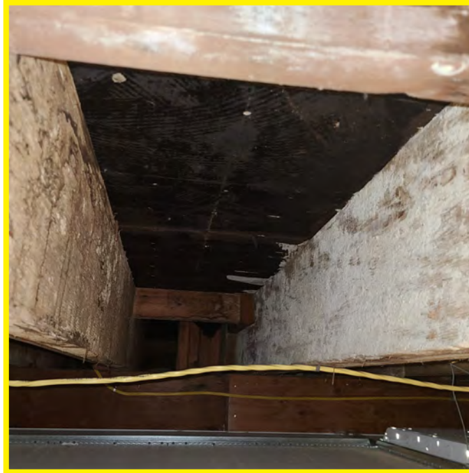
The photo above shows a closer look at the 2nd floor framing elements. Joist bracing or blocking appears to be inadequate. No fire rating is observed. Stuctural framing needs to be inspected by an engineer. Replacement and increased fastening requirements.
