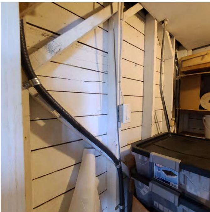
The photo above shows the storage/ janitorial supply room which is accessible in the kitchen area only. Exposed electrical and interior wall structure can be observed.
