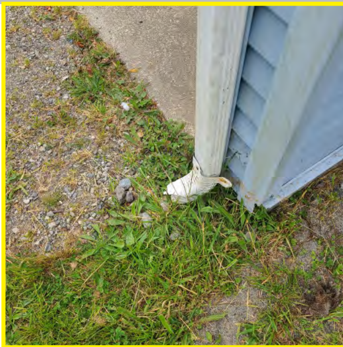
Photo above shows downspouts draining to surface. No splash pads are observed to prevent ground erosion. Ground shows significant organic growth around building in 'non-landscape' areas.
