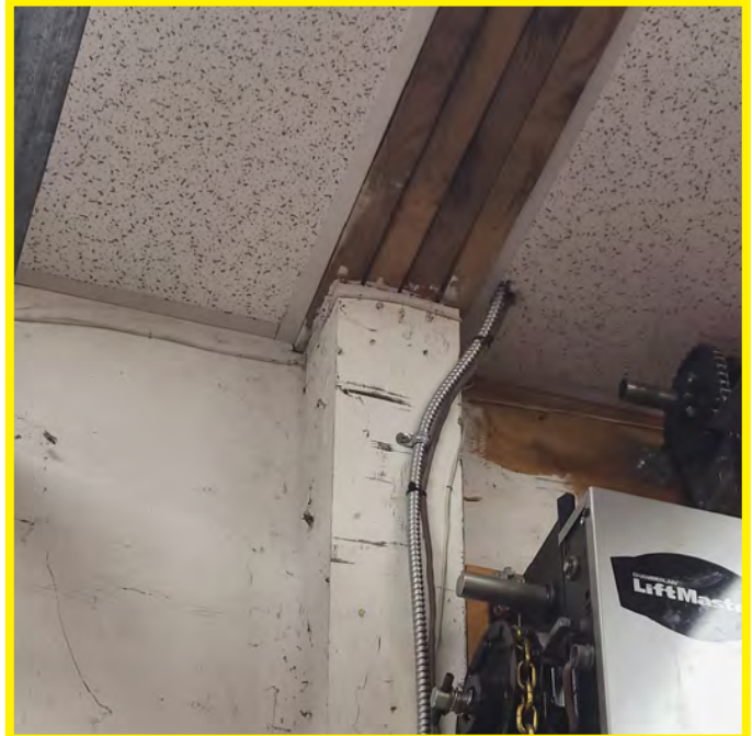
The photo above shows the continuation and support of the structural floor beam member terminating at the front wall location. The size of column is unknown. The column is assumed similar rough-sawn wood. Proper bearing? Lack of fastening. NON-SEISMIC.
