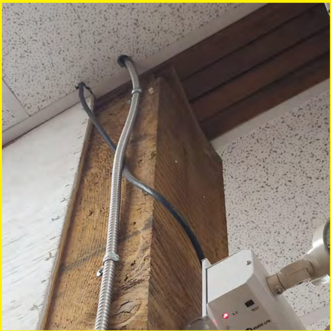
Reference previous photos for further information on photo above. This photo shows another partition wall. Exposed electrical and emergency lighting wiring is observed. The beam above is shimmed and appears to lack appropriate fastening requirement.
