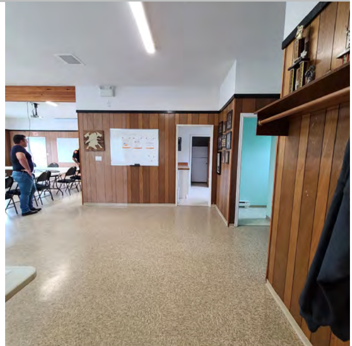
The photo above shows a view of the washrooms, kitchen, and training/ multi-use areas. The flooring and interior aesthetic is outdated.
