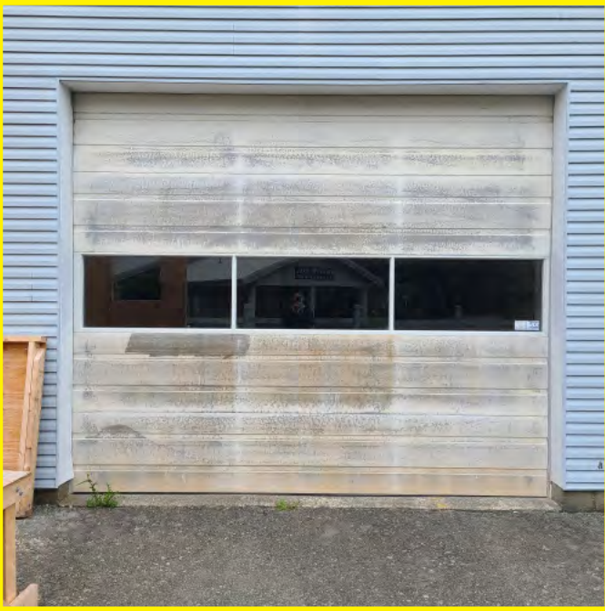
Photo above shows rear overhead door has surpassed its product life cycle. This overhead door may be an acceptable size if used only for access and egress of small equipment.
