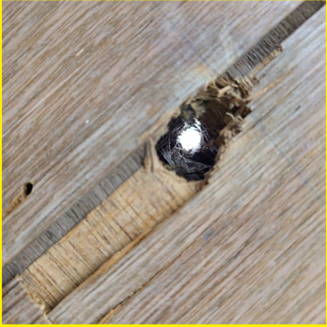
The photo above shows a hole through the complete building envelope. Daylight can be seen from the interior. The building wall assembly does not appear to be acceptable.
