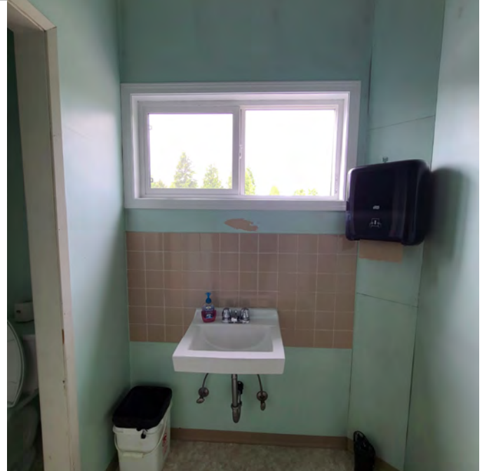
The photo above shows outdated washroom accessories and awkward washroom layouts.
