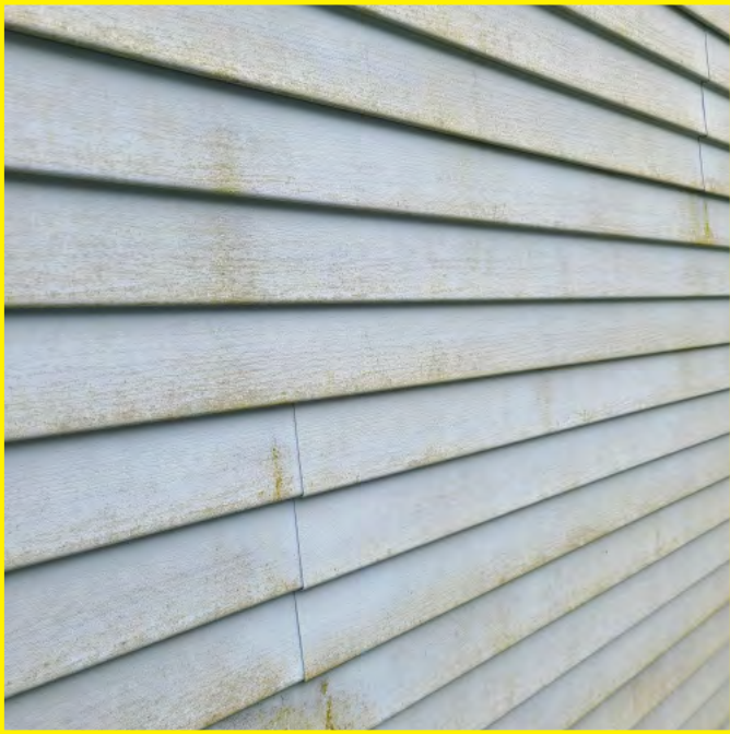
Photo above shows a close up of the exterior vinyl cladding. This material should not be used on a building of this type. Significant signs of weathering are further shown. Exterior cladding should be replaced with a non-combustible material.
