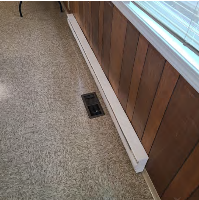
The photo above shows the building heating components.
