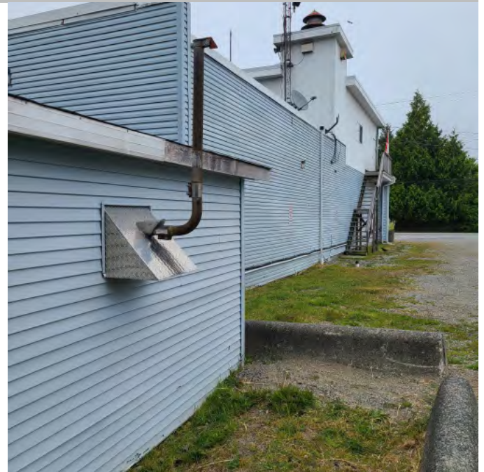
The photo above shows significant organic growth along the building facades. The buildings show outdated architectural and building envelope details. Fascias and flashings are deteriorating.
