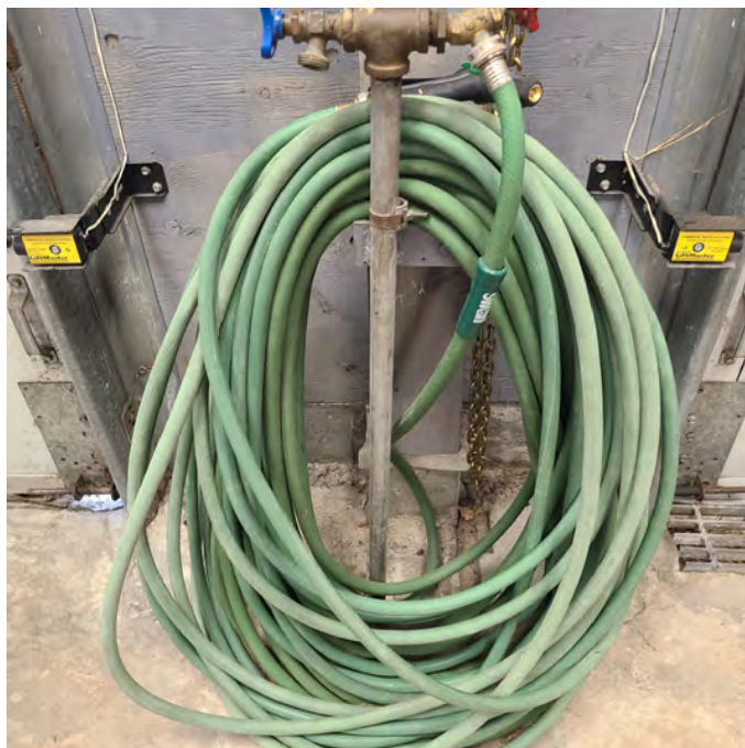
The photo above shows an interior hose bib that is used for vehicle washing. This needs to be relocated and mounted for proper storage.
