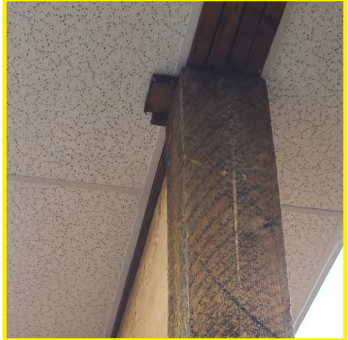
The photo above shows an exposed 4-ply built-up wood beam supporting the floor above. It is assumed these members are continuous over the column support. Proper structural fastening or metal brackets appear completely absent. Shimming is wedged.
