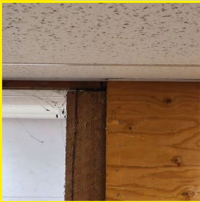
The photo above shows a close up look at one of the interior partition walls. This wall is assumed to be a structural shear wall supporting the floor above. The connections do not appear to be seismically sound.
