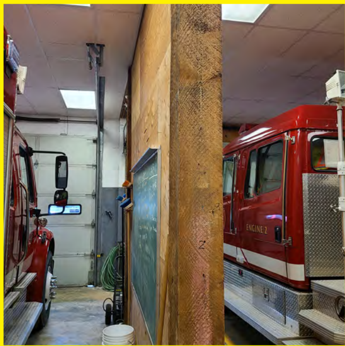
The photo above shows a dividing partition wall between the main truck bays. This wall is comprised of rough-sawn timber columns and plywood sheathing. This wall is assumed to be a structural element. No fire rating protects these elements.
