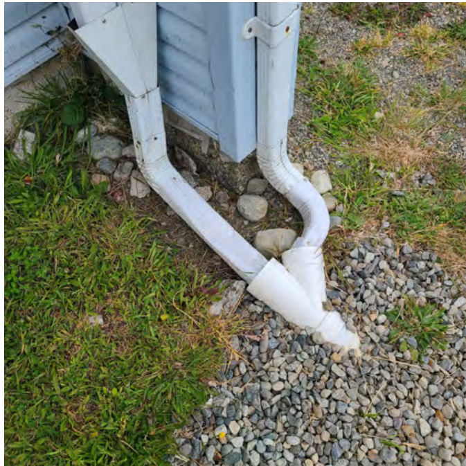
The photo above shows that while SOME perimeter storm drainage is installed, it has not been installed properly and appears to not be installed at the required depth for frost protection. This installation would fail a current building inspection.
