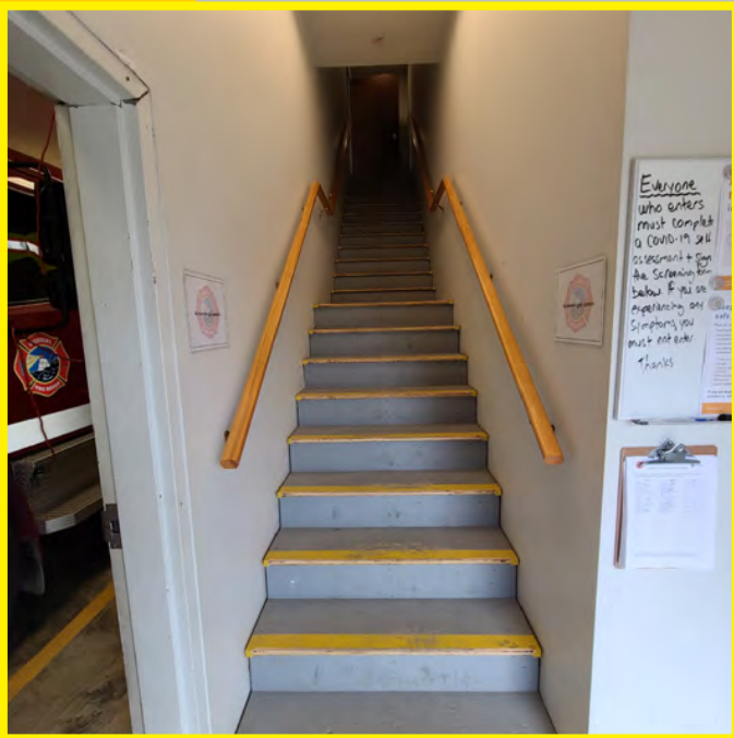
The photo above highlights the stair and handrail issues. The stair treads do have proper nosing but have a steep rise and run and inadequate headroom as required by code. The door frame appears to be poorly installed or unfinished.
