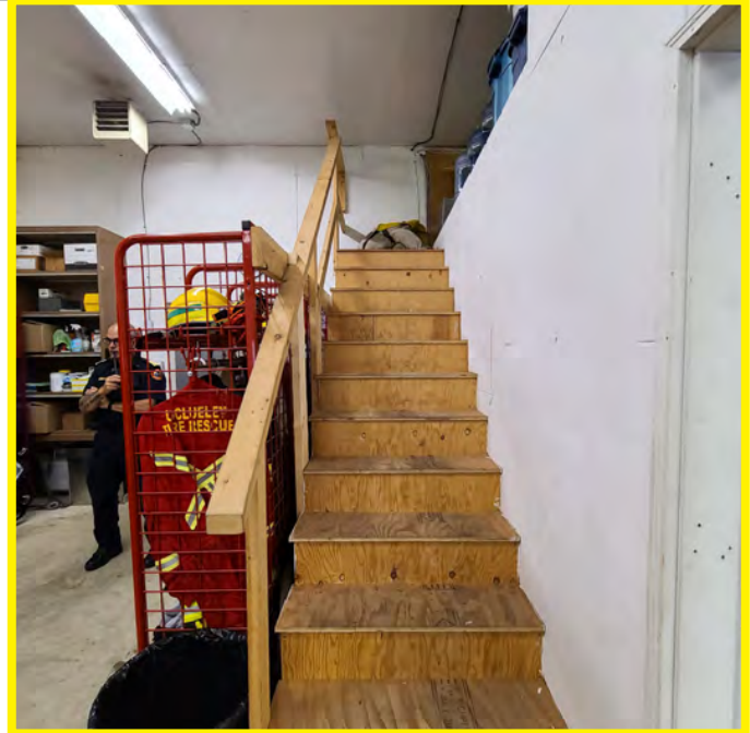
The photo above shows access stairs to the storage mezzanine. The stairs and railing are not built to code. A small unit heater is observed to be mounted to the underside of the ceiling in the gear room.
