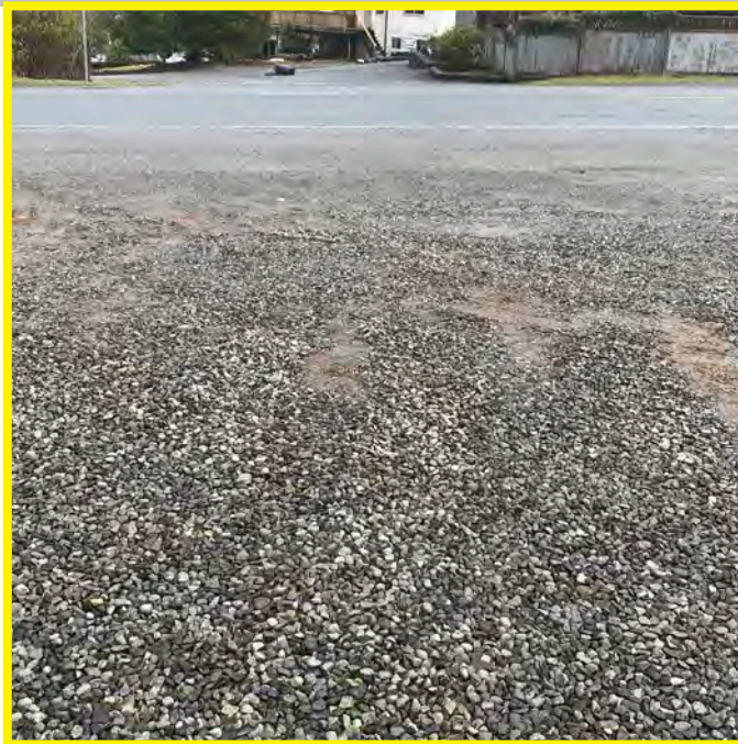
The photo above shows that although most of the site appears generally stable during warm dry months, poor soils conditions and soft spots become visible during the fall and winter months. Geotechnical investigation should be conducted.
