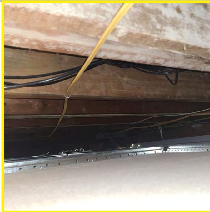
The photo above shows a look above the apparatus bays acoustic ceiling tile finish. The t-bar does not appear to be seismically fastened to the underside of structure. No fire rating is observed. The structure appears to just be dimensionally wood framed.
