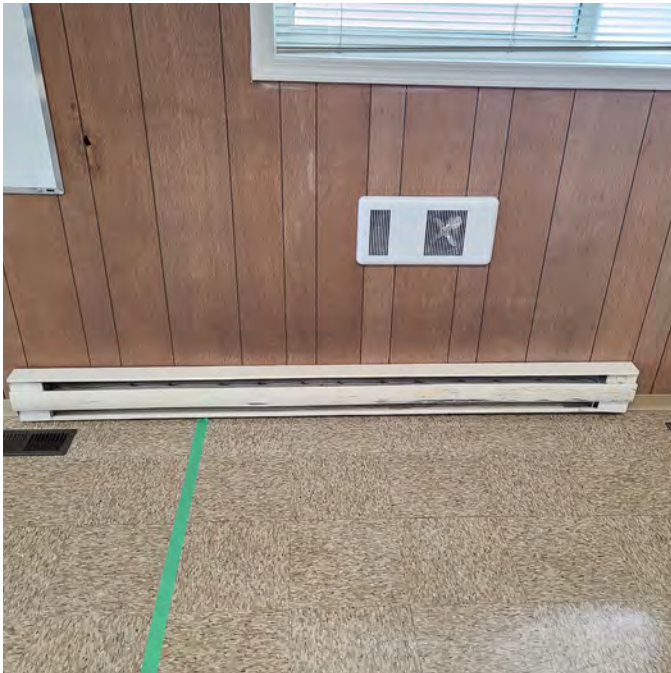
The photo above shows electric baseboard heating and wall register. The photo also shows a closer look at the outdated VCT tile and wall finish.
