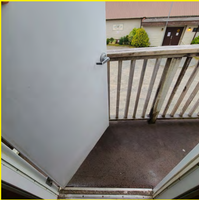
The photo above shows the second floor emergency exit stairs. The door does not have any emergency panic hardware and the door can only open approximately 75 degrees. The railing wood railing is weak and shows signs of significant weathering.
