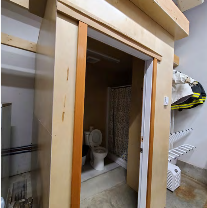
The photo above shows the only available washroom on the main floor. This washroom/ shower room combo is not sufficient for a decontamination room which should be available in the apparatus bays.
