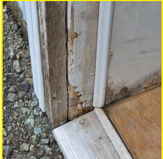
The photo above shows a rotting rear door jamb and interior base of wall near the sill. It is clear that proper door installation details were not followed allowing water leakage into the building envelope. A commercial type door should have been used.
