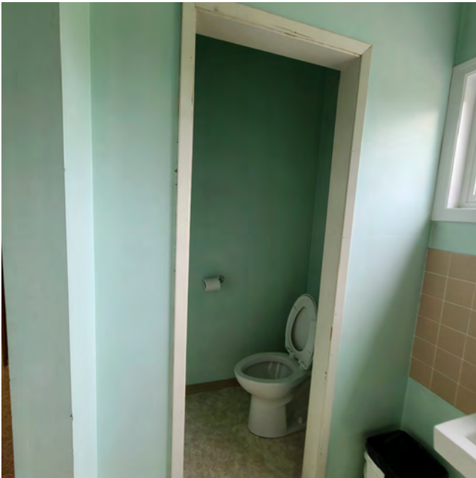
The washrooms are inadequate for the facility uses.
