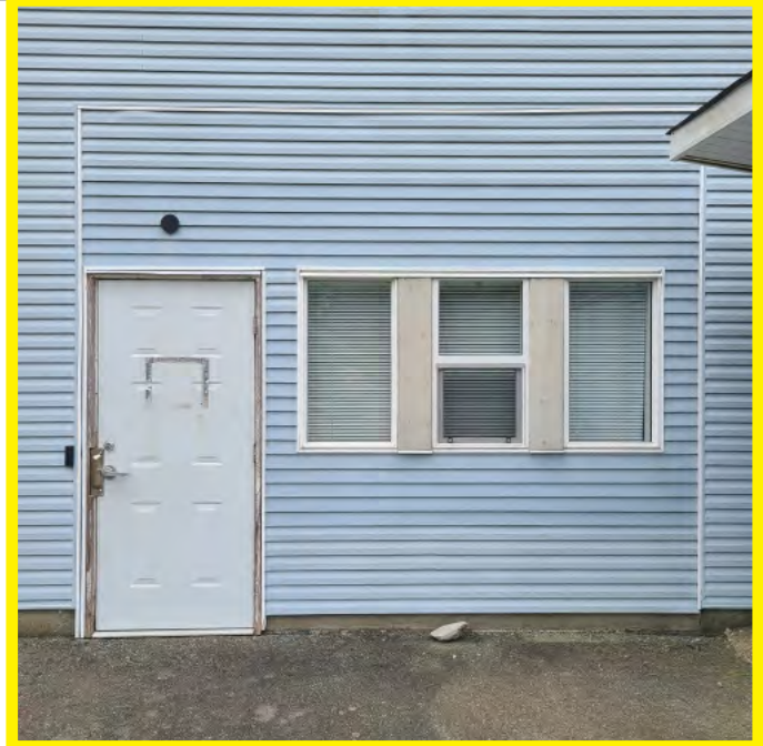
Photo above shows patchwork to building envelope and inadequate window and door details. It is assumed that the building envelope has completely failed and no longer keeps out water from the wall assembly. Windows are old and past product life cycle.
