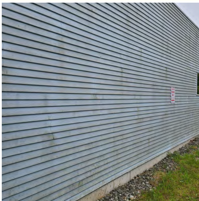
Photo above shows vinyl exterior wall cladding. It is obvious that the vinyl cladding has exceeded its product life cycle and needs to be replaced. Immediate maintenance is required. Significant signs of weathering.
