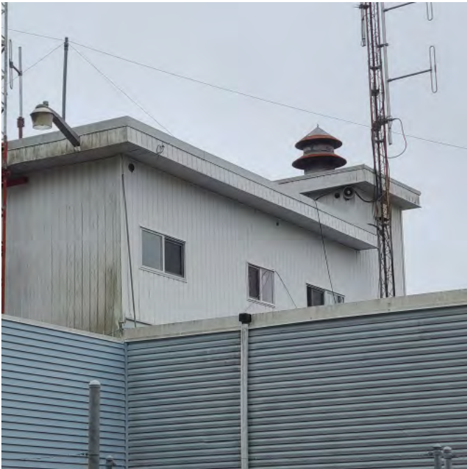
Photo above shows rear of second storage. It is obvious that the building envelope has failed. Roof scuppers require replacement. Exterior mounted equipment needs relocation and proper mounting.
