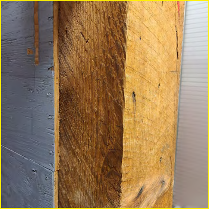
The photo above shows a close up look at the rough-sawn columns and what is assumed to be a shear wall nailing pattern at the edges of the plywood sheathing. The structural adequacy of the columns and acceptability of the nailing cannot be confirmed.
