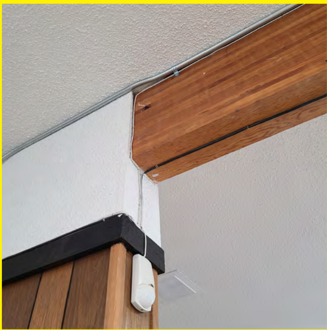
The following photos show elements of the supporting roof structure. A single exposed glulam beam is observed. The bearing and support column is hidden in the wall and cannot be confirmed adequate.
