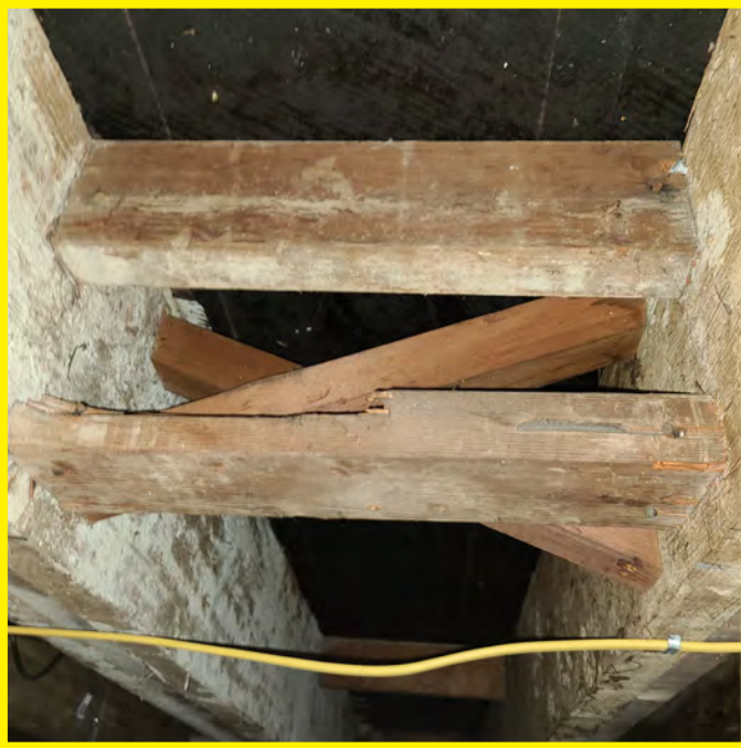
The photo above shows a closer look at the 2nd floor framing elements. These do not appear to be seismically sound. The wood is dry but it not in good condition. The wood has the appearance of used forming material. - structural details needed.
