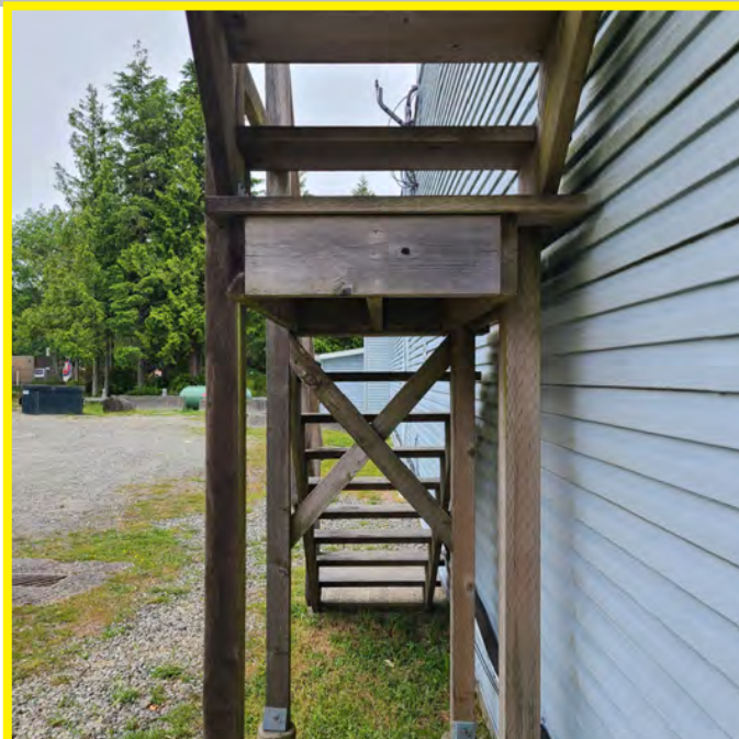
The photo above shows further evidence of the description to the right. The stairs are not properly secured to the building structure.
