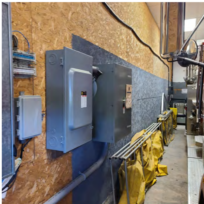
The photo above further shows that movement is limited around all sides of the trucks in the fire hall. Electrical equipment needs relocation to a proper electrical room.
