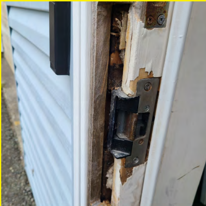
The photo above shows a clear example of building envelope failure at the rear entry door jamb. Rot and deterioration is clearly present and likely is also present within the wall assemblies. The section of rot lessens the security level of this entry point.
