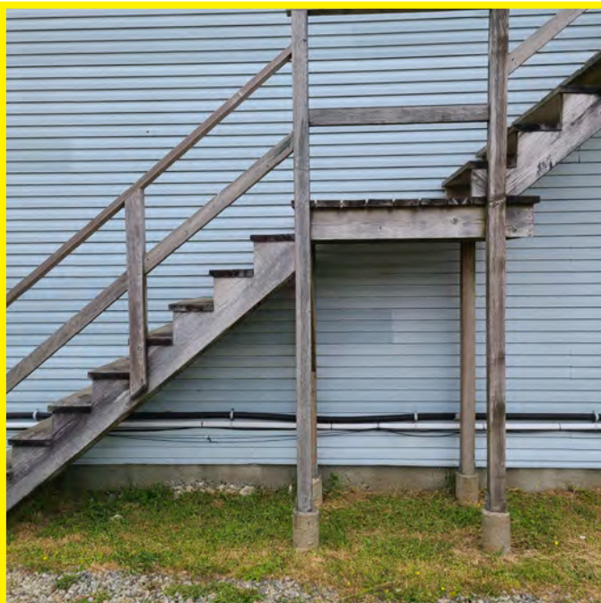
The photo above shows construction of exterior stairs. The staircase is not built to code and is inadequate for use as an emergency exit.
