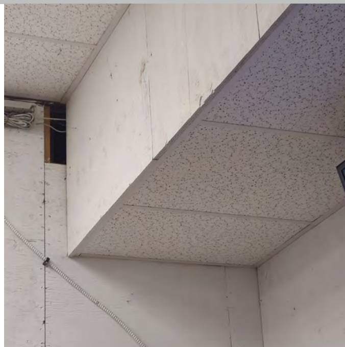
The photo above shows the poor patchwork condition of the interior wall 'finishes' and surface mounted electrical. No fire rated material is observed around bulkhead areas.
