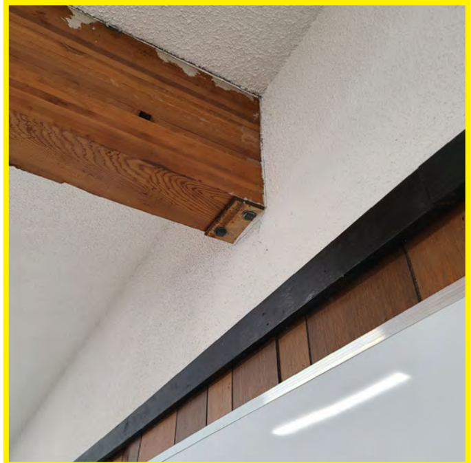
The photo above shows the glulam beam support at the front exterior wall. The beam is fastened to a metal bracket. The integrity and adequacy of this connection cannot be confirmed. It does not appear seismically sound.
