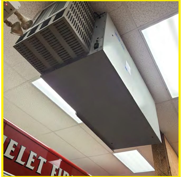
The photo above shows a single air scrubber unit centrally hung over the main apparatus bays. Efficacy cannot or proper operation cannot be confirmed to meet WCB standards with respect to controlling carbon monoxide levels from truck exhaust.
