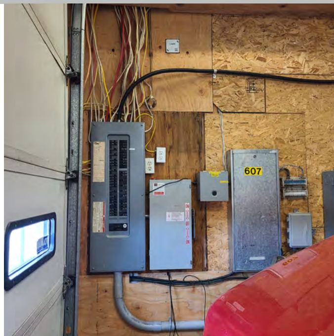
The photo above shows the surface mounted electrical room positioned within the apparatus bay area. This should be within a dedicated fire rated electrical room. The wiring and fuse switches are exposed and are very near to the door.
