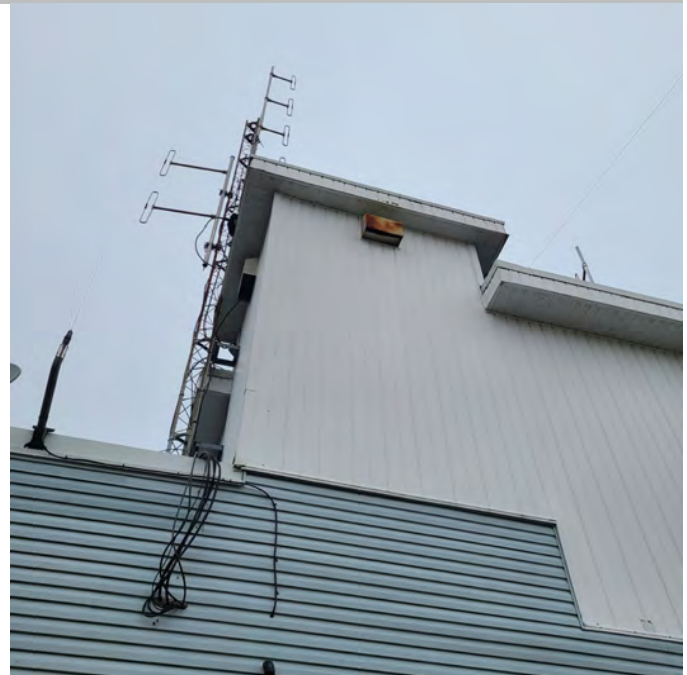
The photo above shows poorly sealed wall penetrations and cladding details. These areas are prone to weather intrusion. Building envelope leaks lead to rot, mold growth, health hazards, and energy performance loss.
