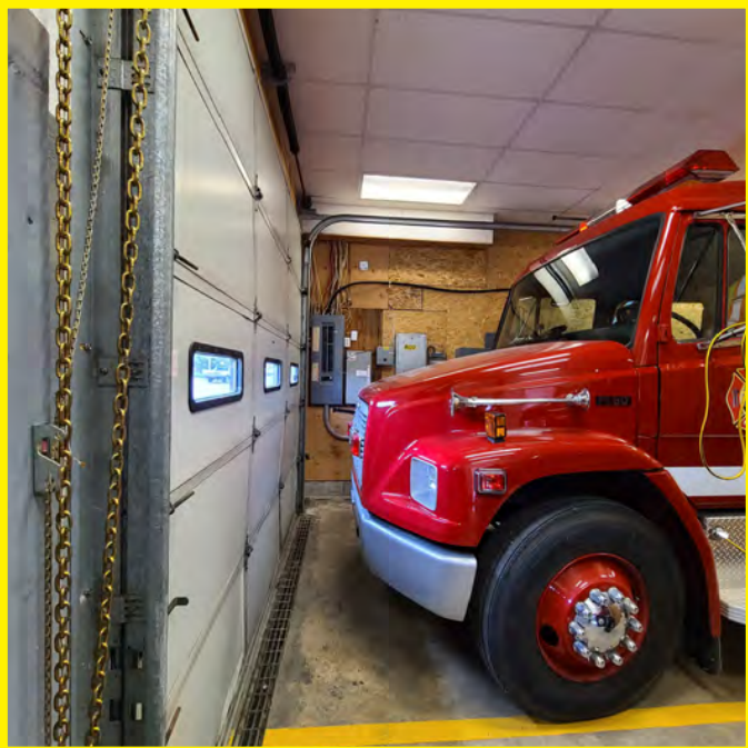
The photo above highlights a number of major issues with the existing Fire Hall that further stress the need for an A&R or new Fire Hall to be constructed: OH door/ drainage, electrical issues/ fire hazards, there is NO ROOM for an aerial truck of adequate walking rm.
