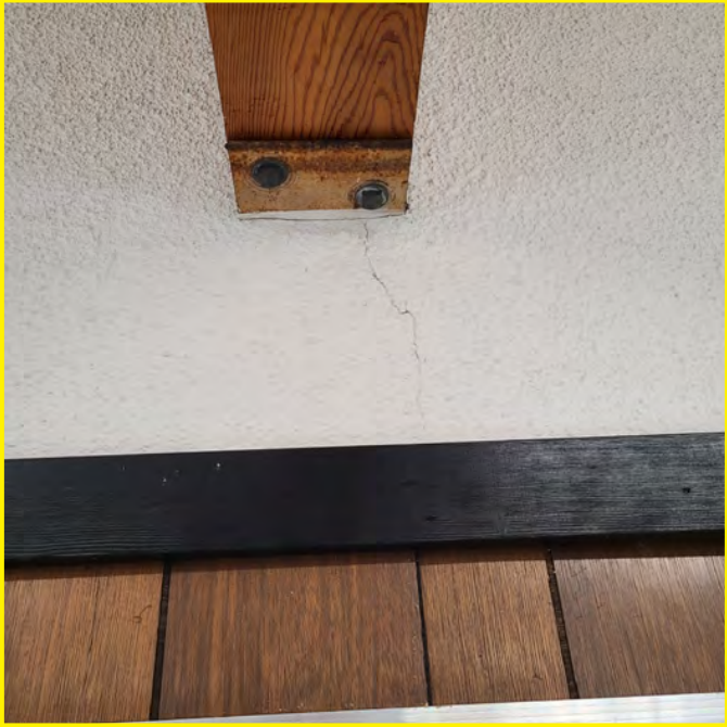
The photo above shows drywall cracking below the glulam beam which indicates building movement and/ or settlement.
