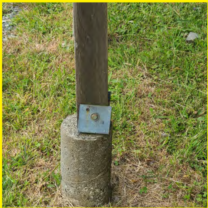
The photo above shows the stairs structural support is inadequately and improperly installed. This detail will cause eventual rot even to pressure treated wood materials. Proper installation and structural fastening is required for life safety areas.
