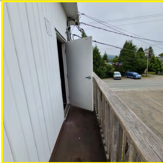
The photo above shows a number of building code and life safety concerns. This exit stair is unsafe for use. The railing is not secure, the door does not open fully, there is no door panic hardware for exiting, the landing is deteriorating, the overhead power lines to the building are not placed safety or neatly, etc..
