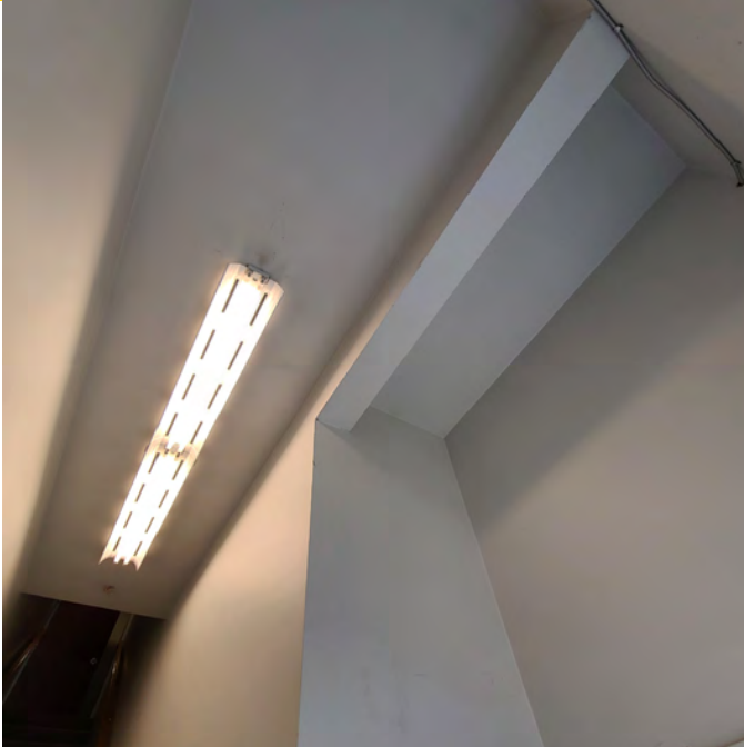
The photo above shows a look at the main entry ceiling and stairwell. One surface mounted light is observed and a supporting beam. The fire rating or structural elements cannot be confirmed.
