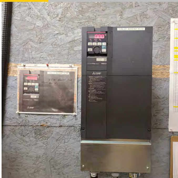
The photo above shows surface mounted equipment controls and surface mounted wiring again a painted OSB wall finish.
