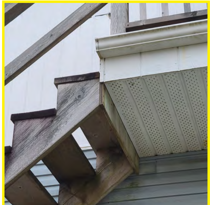
The photo above shows that the stair is not structurally safe. The stairs are deteriorating and should not be used. A small exterior gutter is observed.
