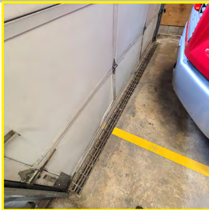
The above photo shows two main areas of concern: 1- improperly positioned undersized trench drain 2- undersized apparatus bays
