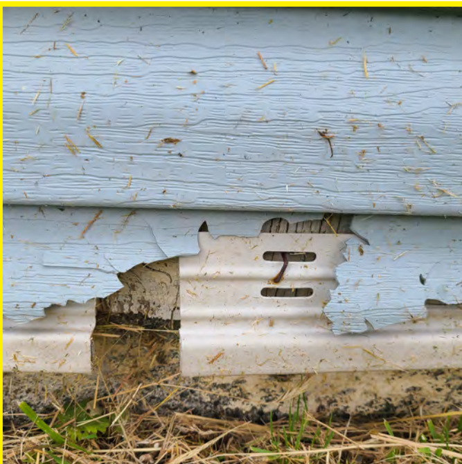
Photo 'A' above shows one example of complete building envelope failure. The vinyl cladding has long passed its product life cycle and is brittle and crumbling. This residential style product is combustible and not suitable for this application.
