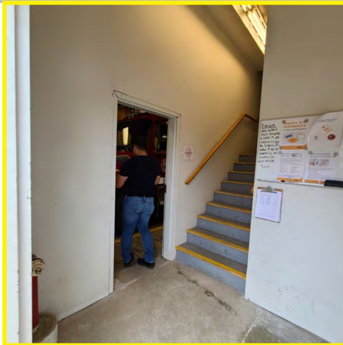
The photo above shows the existing condition of the bare concrete flooring. No concrete sealer appears present or has worn away. The areas of addition are seen. The fire rating of this exit stairwell cannot be confirmed adequate.
