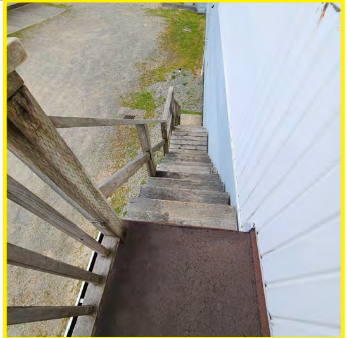
The photo above shows a view from the exterior exit stair landing to the ground. The landing surface is deteriorating and narrow. The hand rail is not of an acceptable design. NOT TO CODE/ unsafe for use.
