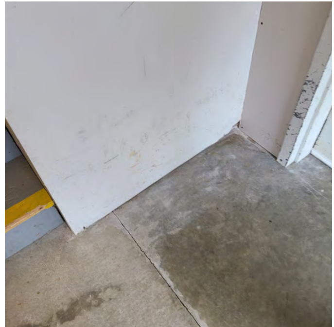
The photo above shows the condition of the main entry concrete slab, walls, and door frames. Maintenance is needed. This photo provides a closer look at the plywood stairs and nosing.
