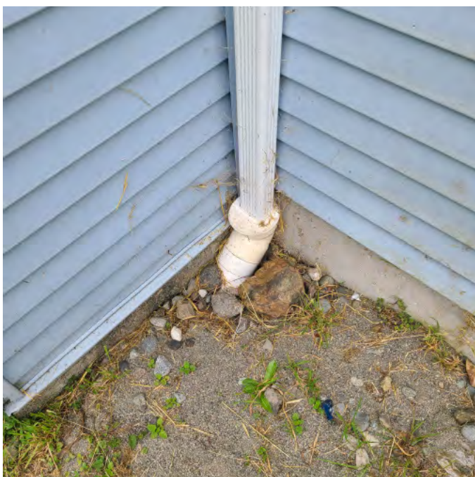
Photo above shows that a perimeter storm water management system is present. The connection appears to be shallow depth. Ground appears unstable due to erosion and organic growth.
