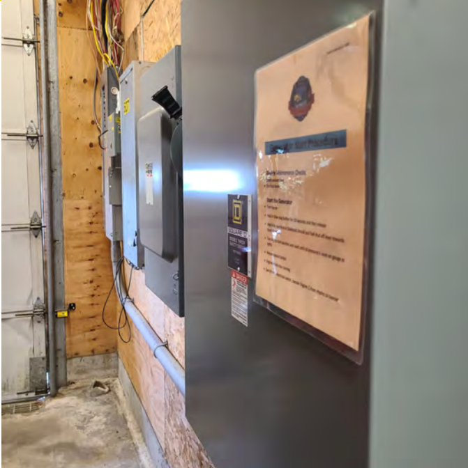
See previous photo notes. Additionally, daylight can be seen along the edges of the overhead door resulting in significant energy loss.
