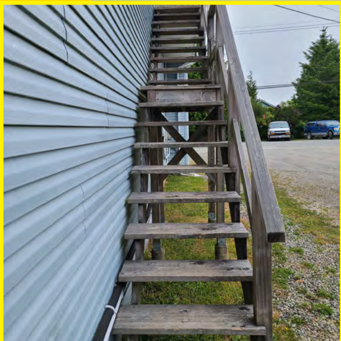
The photo above shows exterior mounted electrical conduit along the vinyl clad wall face. This conduit should be protected. The stairs show significant signs of weathering. The steps and railing are not to building code standards and are loose.
