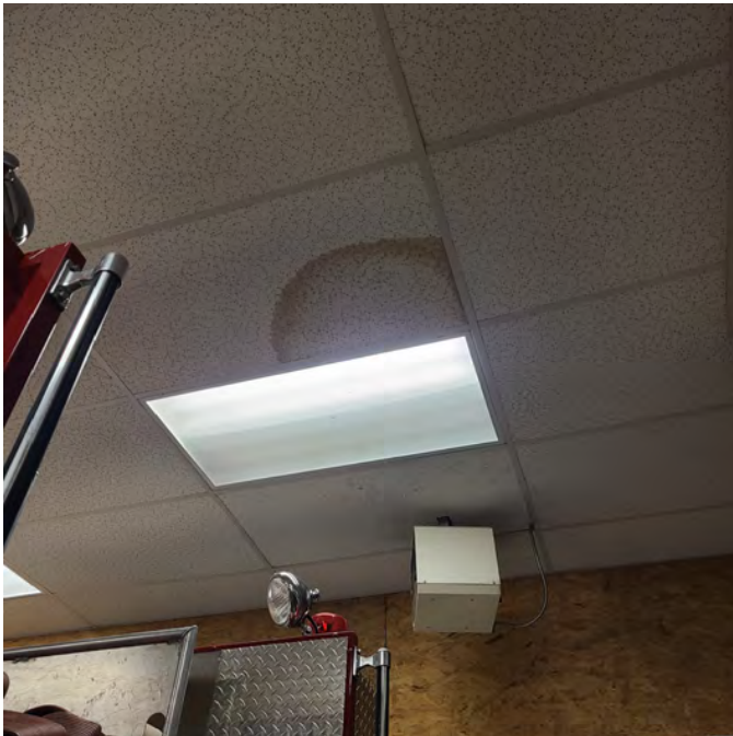
The photo above shows evidence of a previous water leak and subsequent water damage to the ceiling finish. It is assumed this did not cause any structural damage. A small unit heater is hung from the ceiling space and does not appear adequate for the space.
