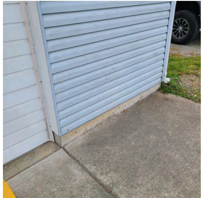
The photo above shows OH door weather protection detail issues. Water may enter the apparatus bays during major rainfall or significant wind driven rainfall events with inadequate sloping and lack of slab drainage.
