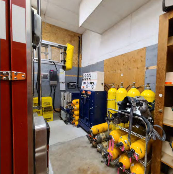
The photo above shows the SCBA and compressor station. The fill station is positioned at the rear of the apparatus bay and has potential for exhaust contamination. Functionality and movement in this area is very limited due to the small space.
