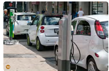
Electric vehicle charging stations
