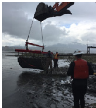
Crews place concrete mats over newly installed conduits (ducts) in the intertidal zone on Protection Island.
