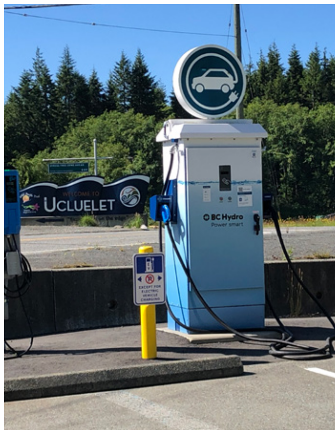
Electric vehicle charging station at the Tofino/Ucluelet junction.
