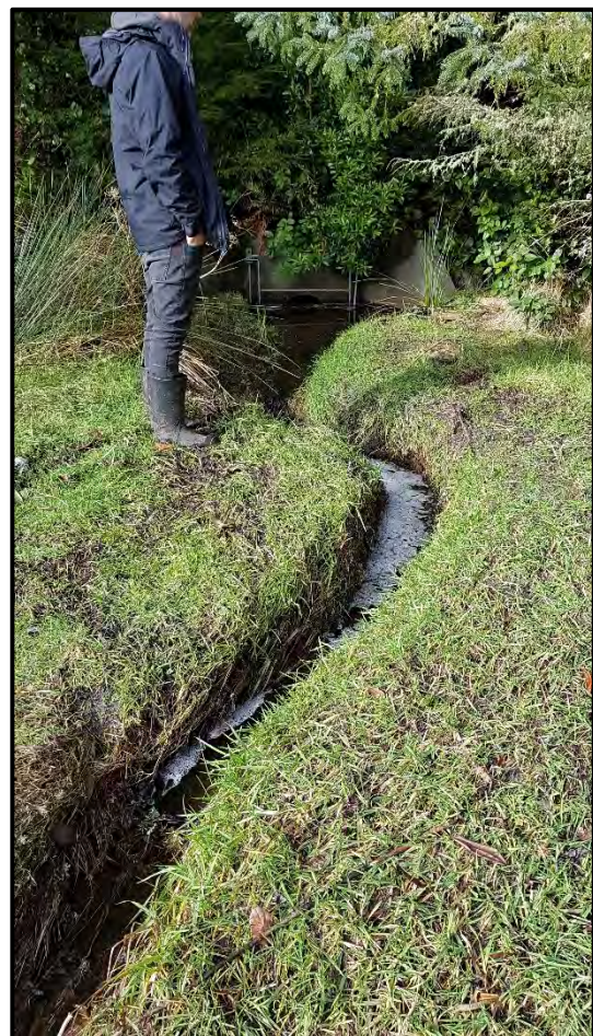
View of drainage/ creek outlet with the ocean 300m away from where it started at the top of the ravine.
