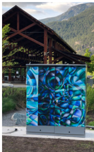
Example of a decorative wrap on our pad-mounted equipment.
