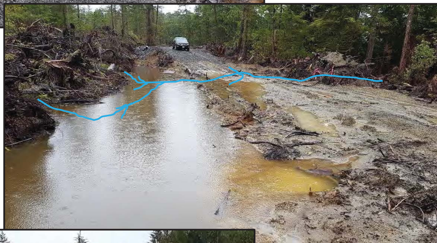
Photo 8: Impacted drainage. Engineer to complete Stormwater management plan for site.
