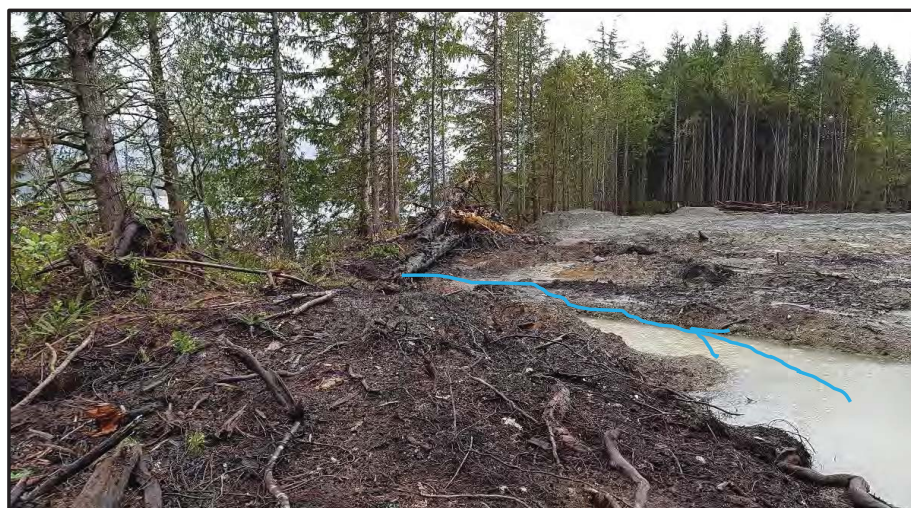
Photo 10: Clearer section of site within 30m foreshore buffer. Riparian buffer to be re-established.
