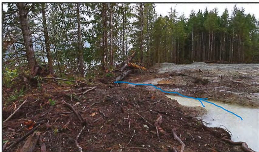
Photo 10: Clearer section of site within 30m foreshore buffer. Riparian buffer to be re-established.
