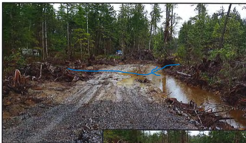
Photo 7: View on opposite side of road alignment in campground area. Clearing went through lower part of drainage.
