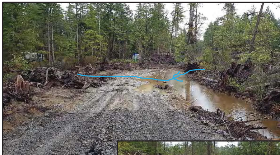
Photo 7: View on opposite side of road alignment in campground area. Clearing went through lower part of drainage.
