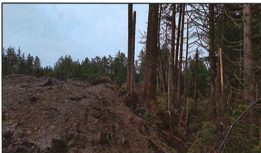
Photo 11: Stockpiled soil burying the base of some trees in 30m foreshore DPA needs to be removed.
