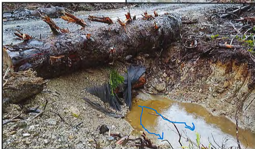
Photo 3: View of Stream 1 and stringer log bridge. Bridge to be removed and replaced. 6" flow clearance
